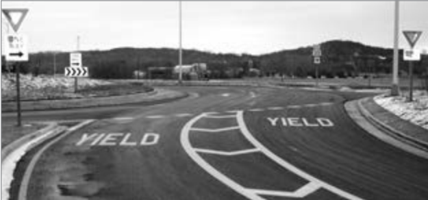
Figure 2-16b: Occasional entry with double white lines separating entry lanes. STH 35 and Hanley Road near Hudson.
